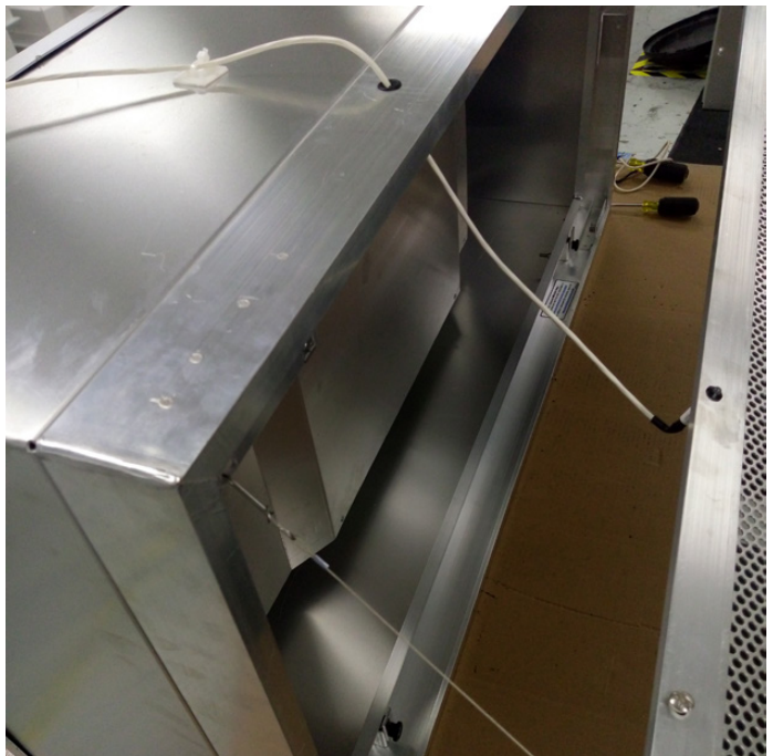
FIGURE 8 - ZIP-TIED LED WIRE WITH PROPER SLACK ▼
